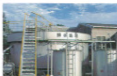
排水処理施設 Drainage Treatment Plant
