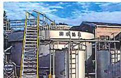
排水処理施設 Drainage Treatment Plant
