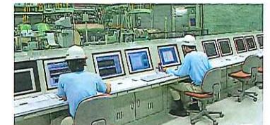
N-1号抄紙機制御室 Control Room of Paper-Making Machine N-1
