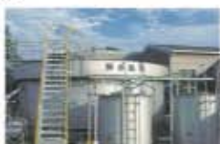
排水処理設備 Drainage Treatment Plant
